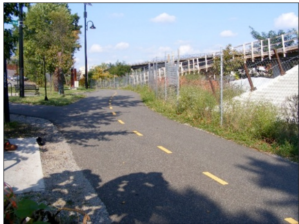
The Metropolitan Branch Trail and Rhode Island Avenue Pedestrian Bridge to the Metrorail platform (in construction). Image Source: Brent Beane on behalf of ULI Washington.
